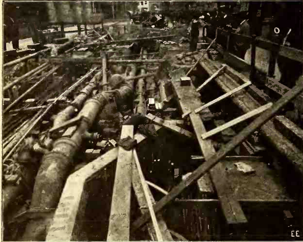
Showing Vast Net Work of Electric Gas, Water and Steam Conductors in a New York City Street Exposed During Building of New Subway.
